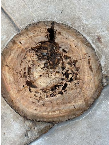
Old wood pole showing The rotting interior
